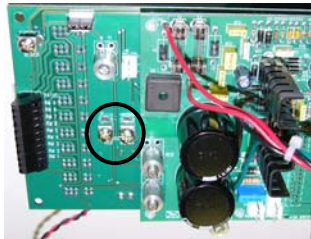
Figure 15 - Door Station Connections
